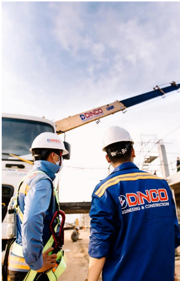
Figure 2. Vietnamese engineers oversee progress at a construction site. Source: DINCO Engineering & Construction
